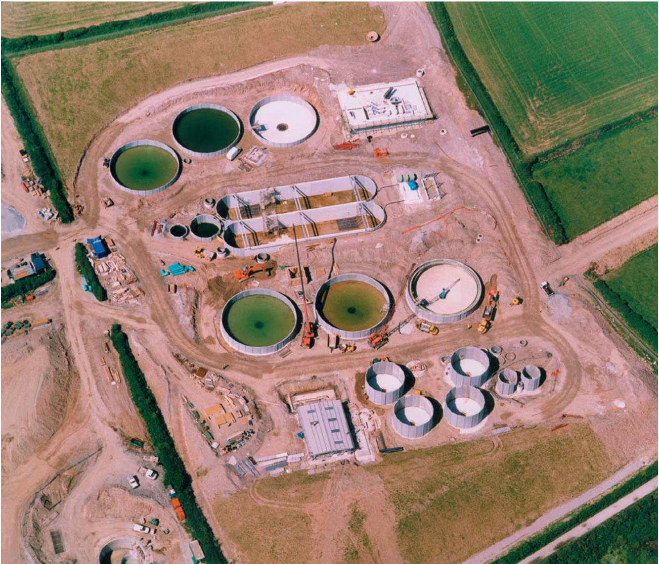
Camborne STW under construction 2001 (photo:: Still Imaging, Chudleigh , Devon; courtesy S.W. Water)
