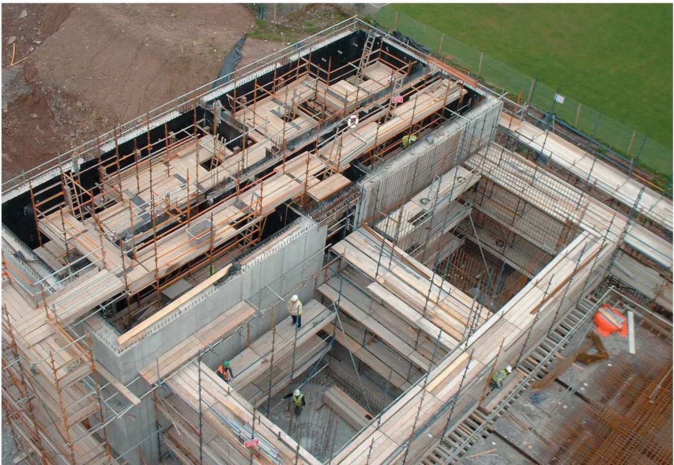
Aerial view of header chamber under construction (courtesy E G Pettit & Company )
